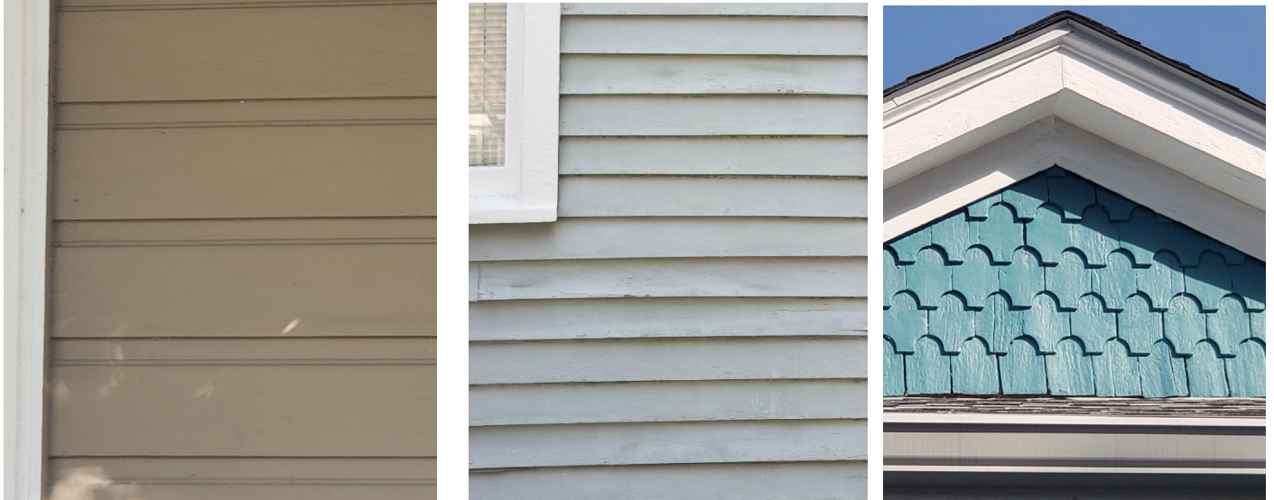
Figure 15: Examples of various types of wooden siding - drop siding (L), clapboards (center), and decorative shingles (R).
