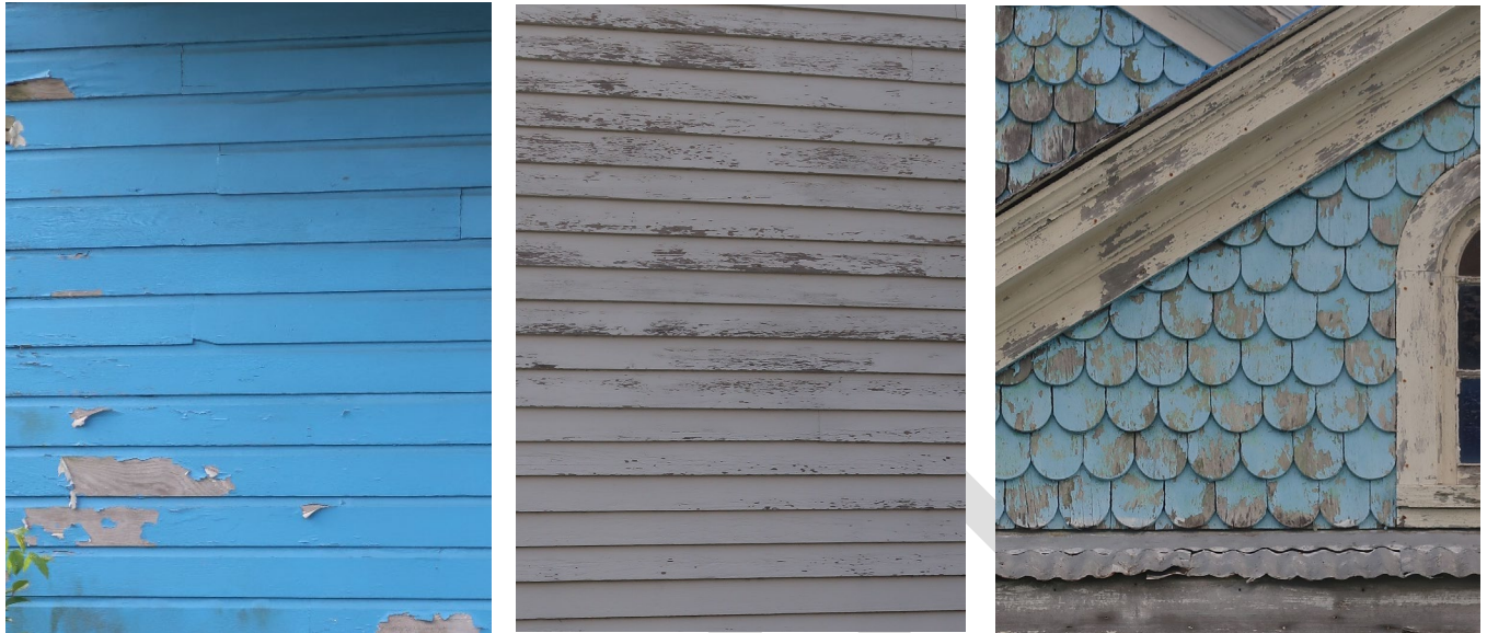
Figure 17: Examples of various types of wooden siding - drop siding (L), clapboards (center), and fishscale shingles (R).
