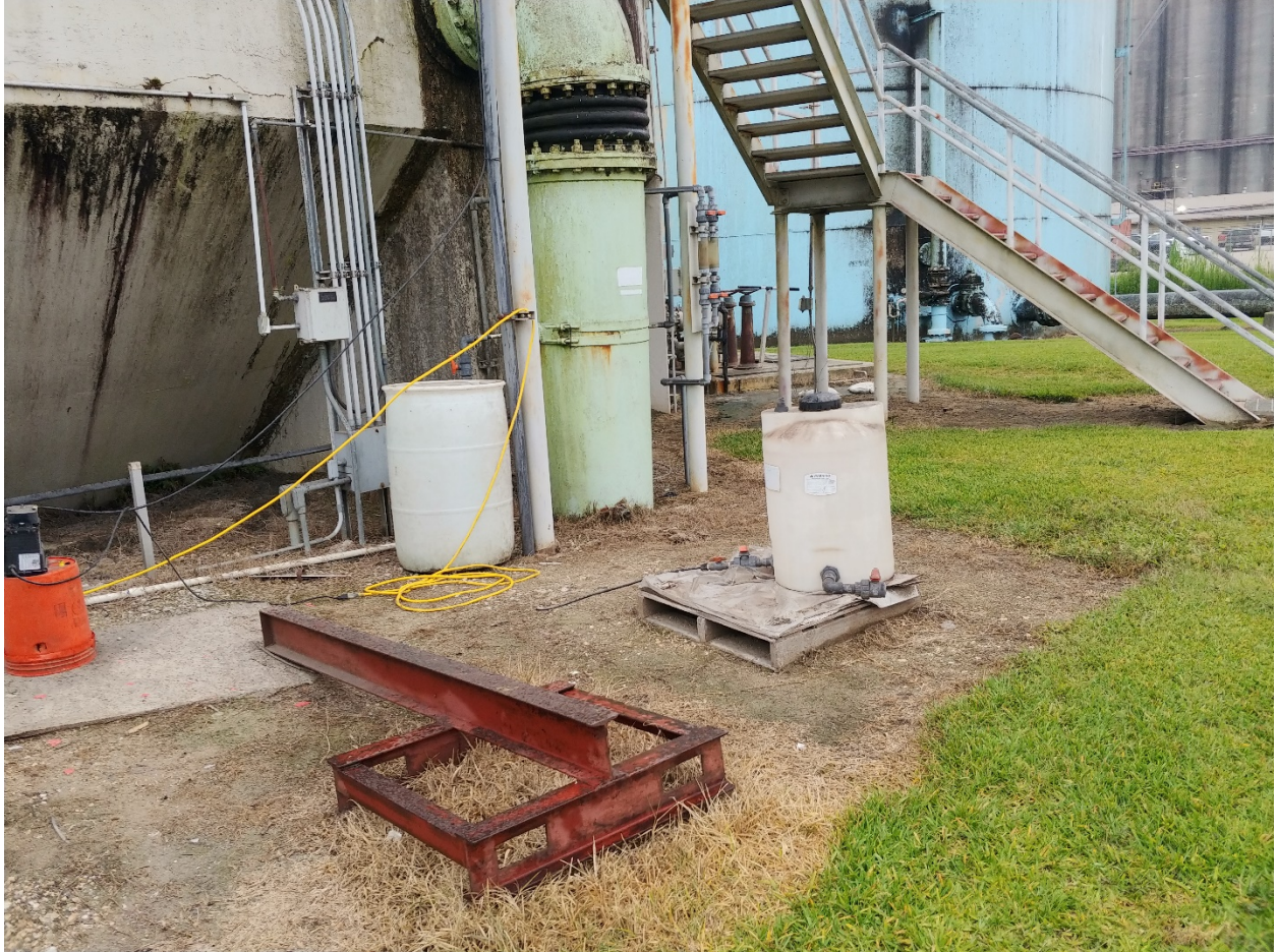
miscellaneous drums and day tanks
