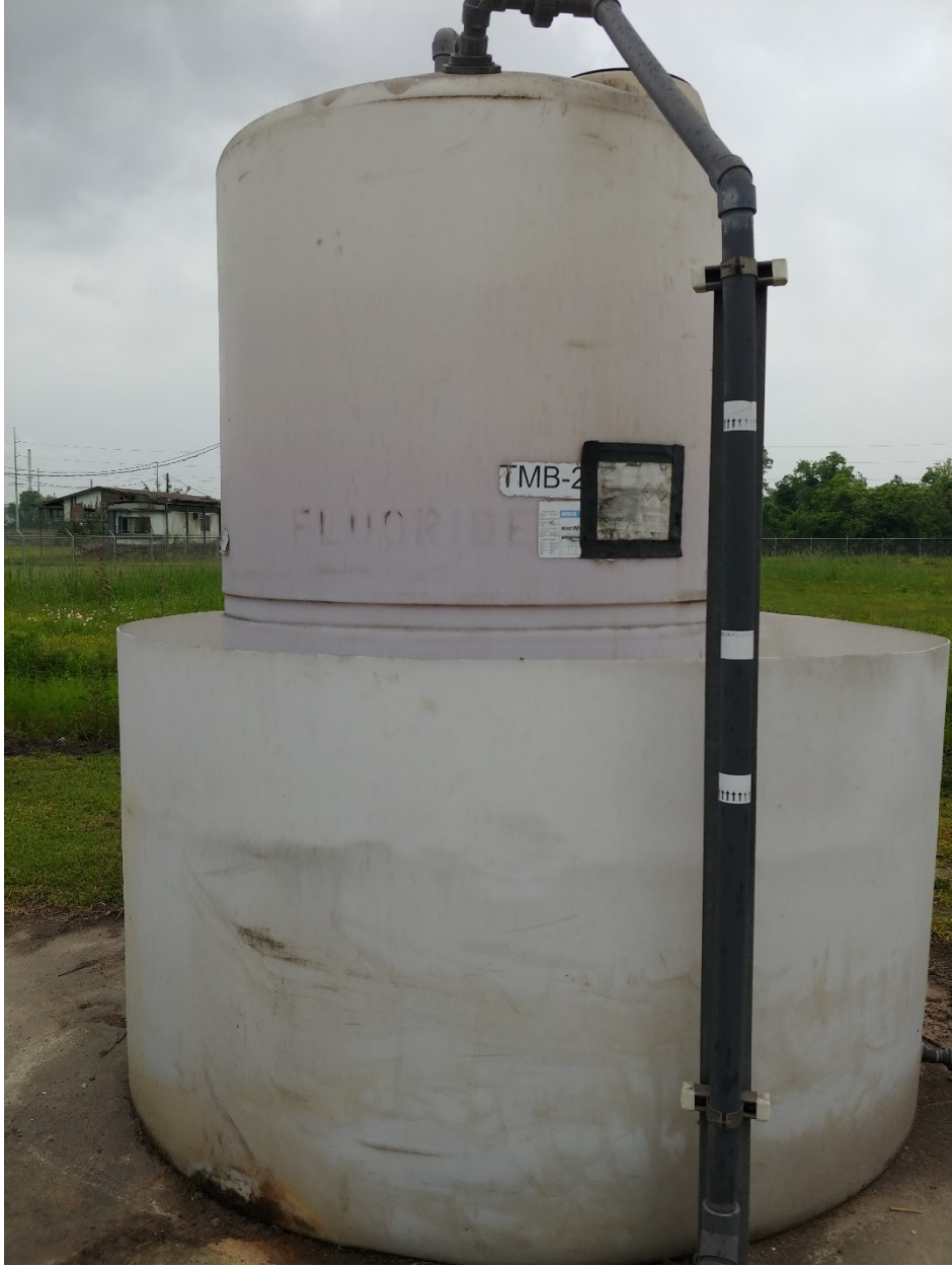
unused fluoride tank
