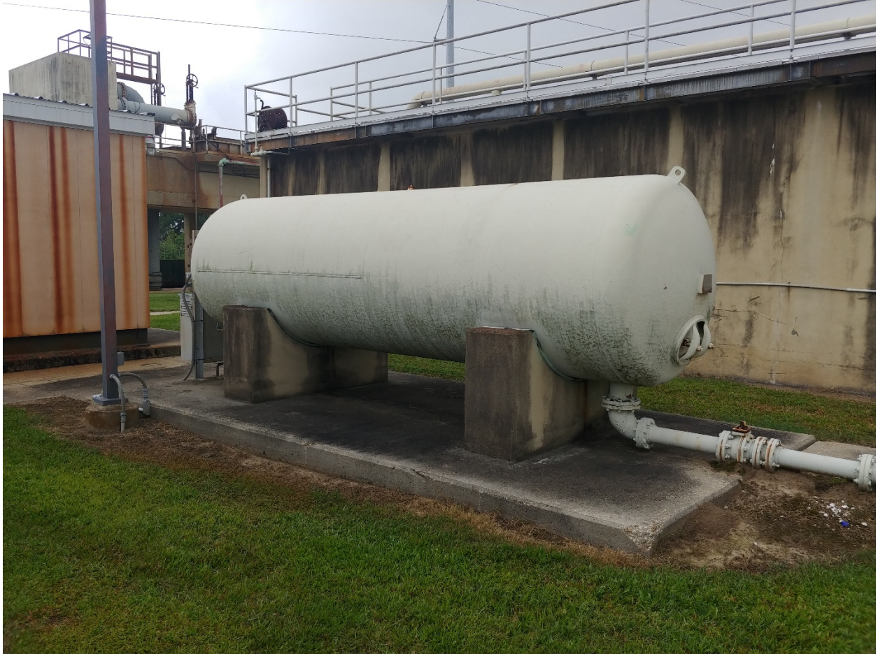
unused process water tank
