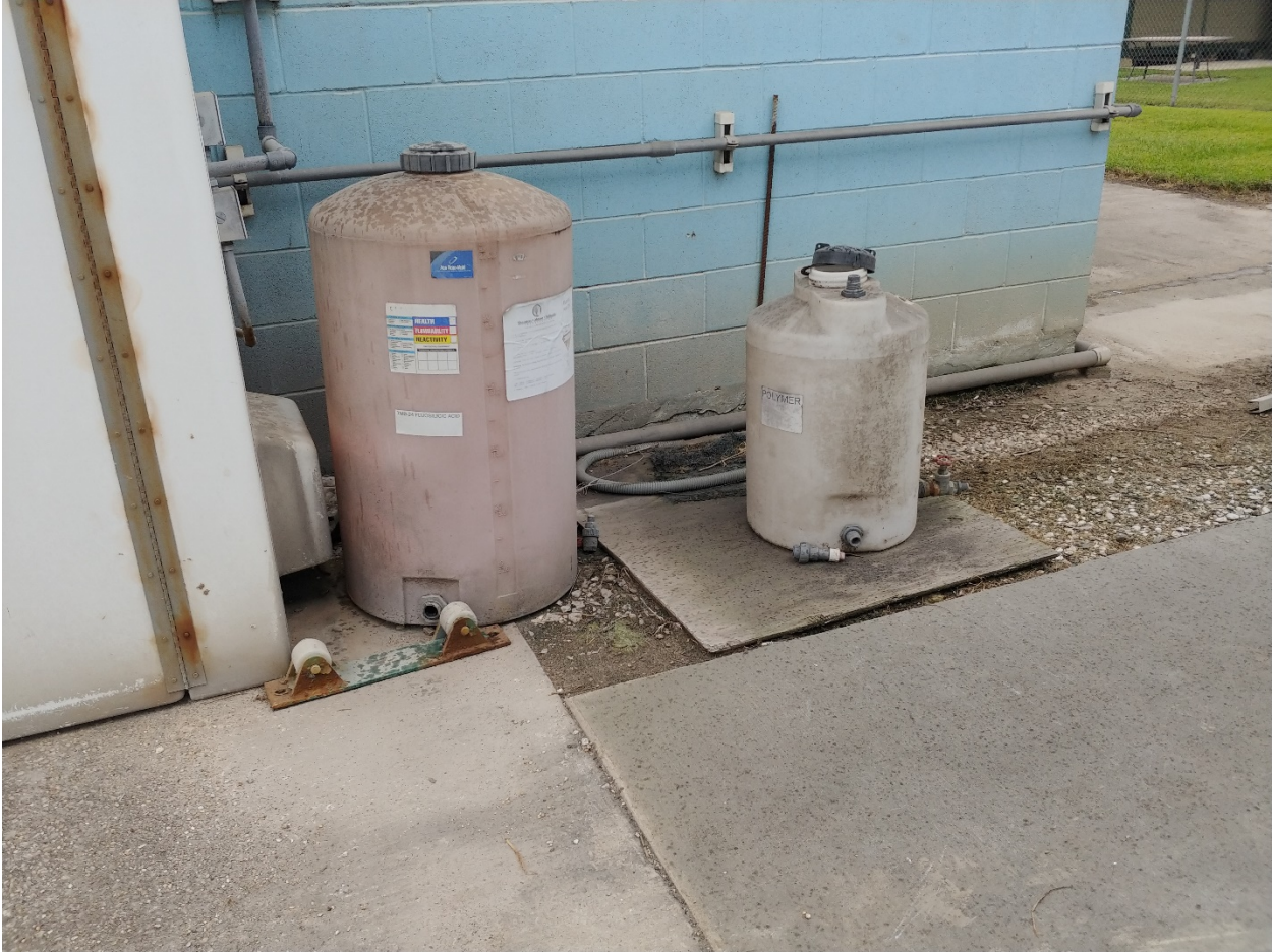
unused day tanks
