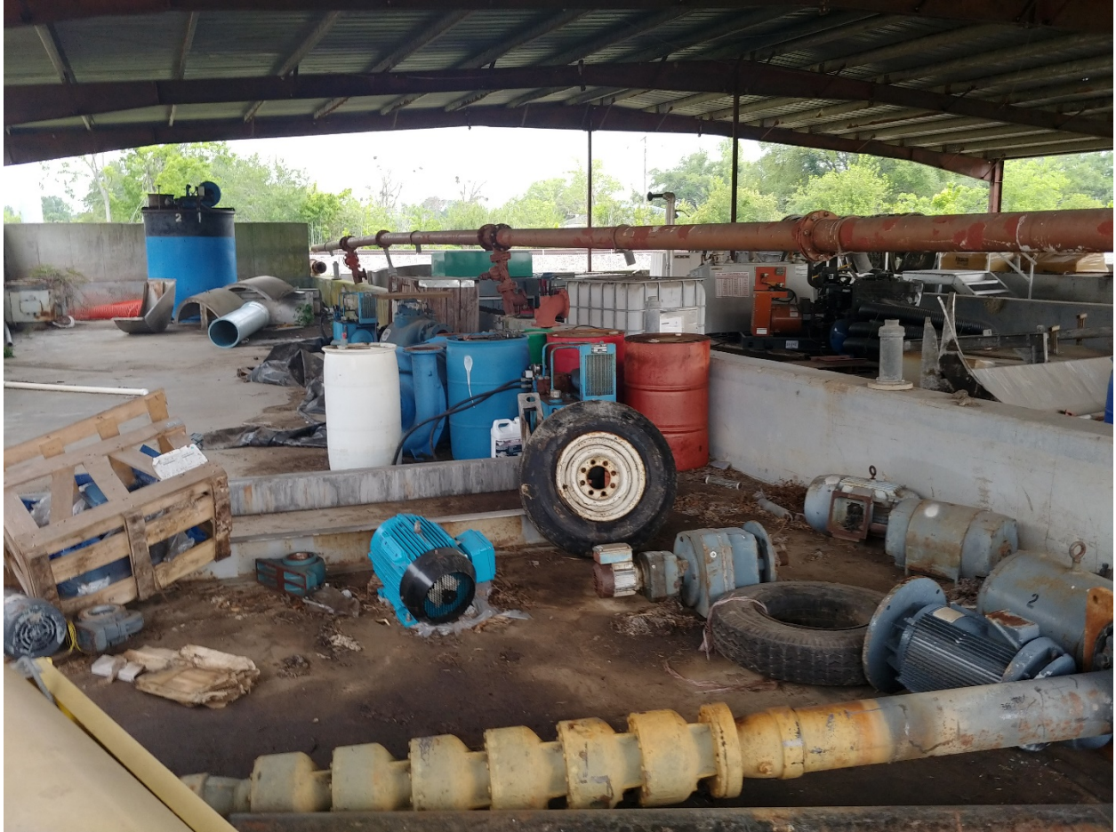
oil drums stored on drying beds; protected from weather, but housekeeping is needed
