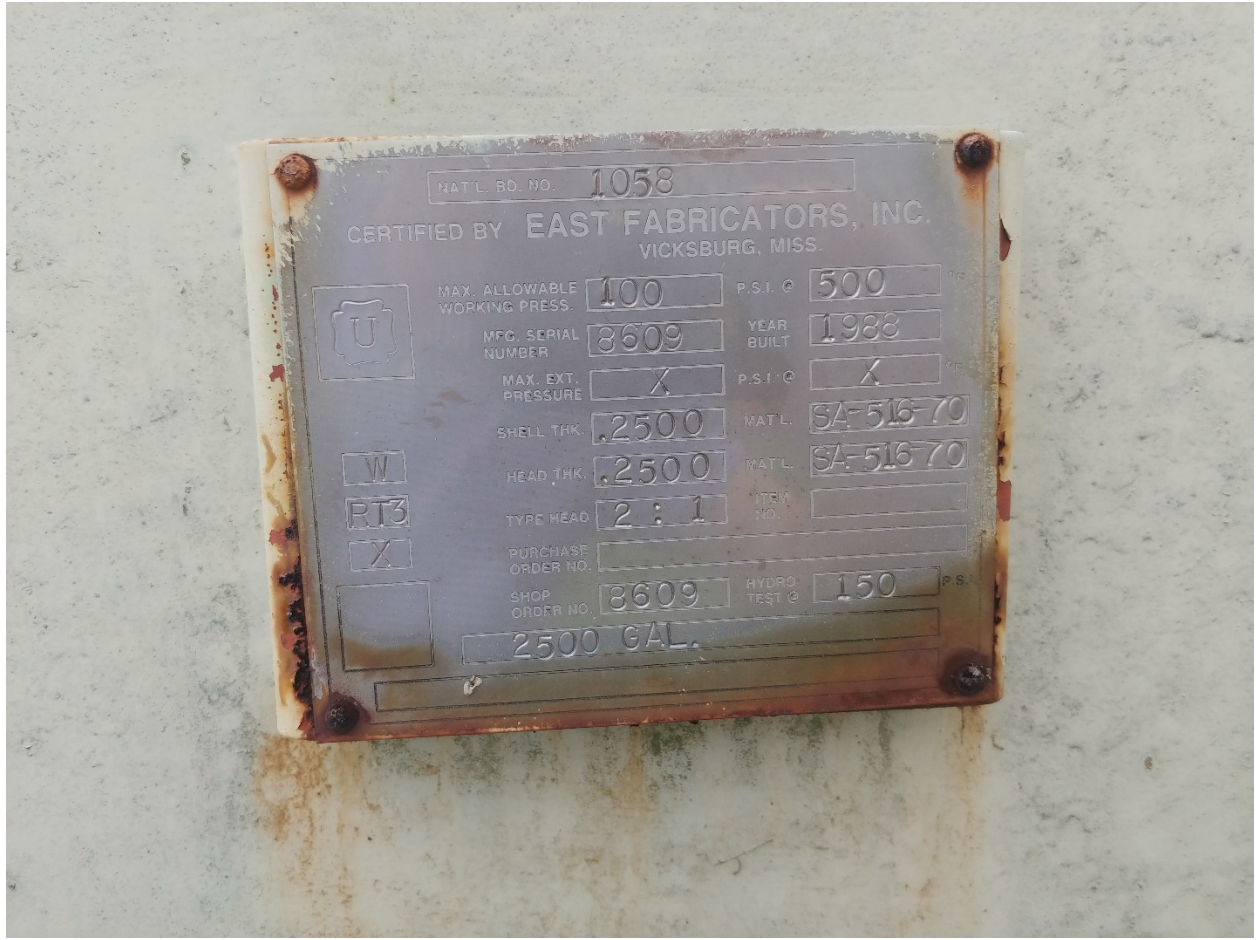
unused process water tank
