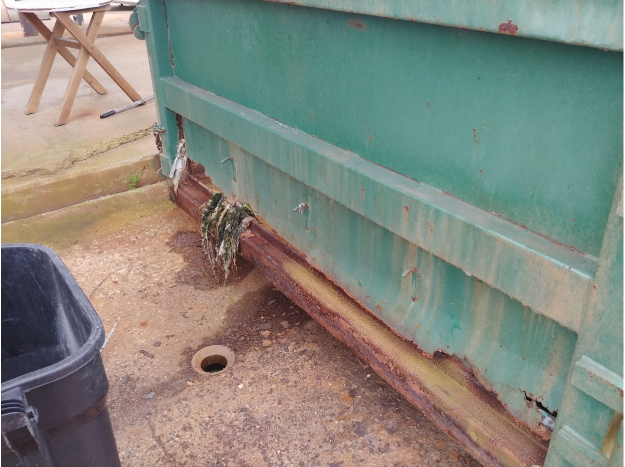
unused damaged rolloff box; drains to headworks
