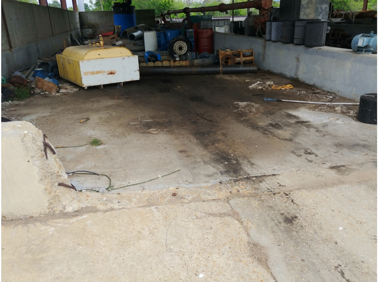
unused diesel tank stored on drying beds
