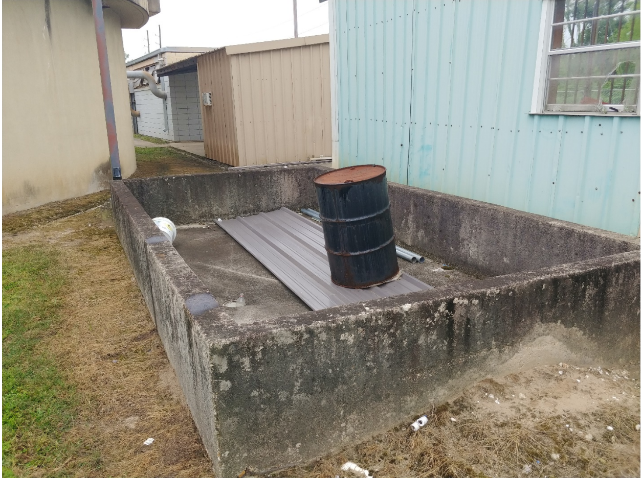
drum storage in concrete containment; unknown where interior drain discharges or if valve is present
