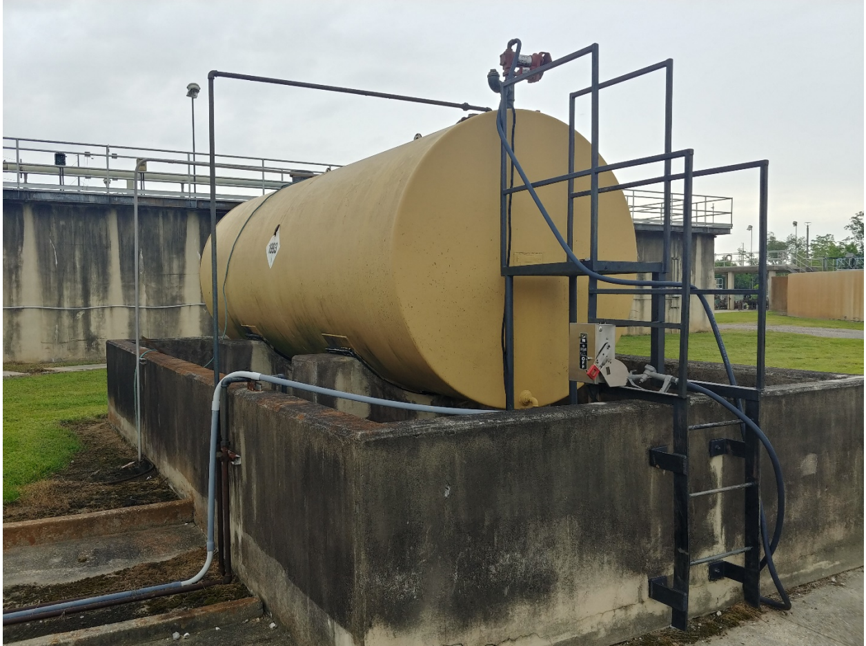
5,000 gallon diesel tank
