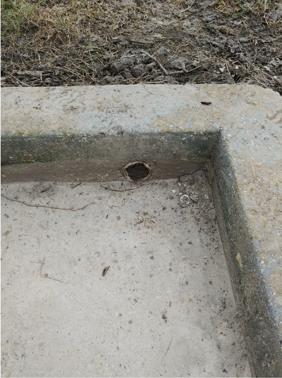
drain for diesel tank
