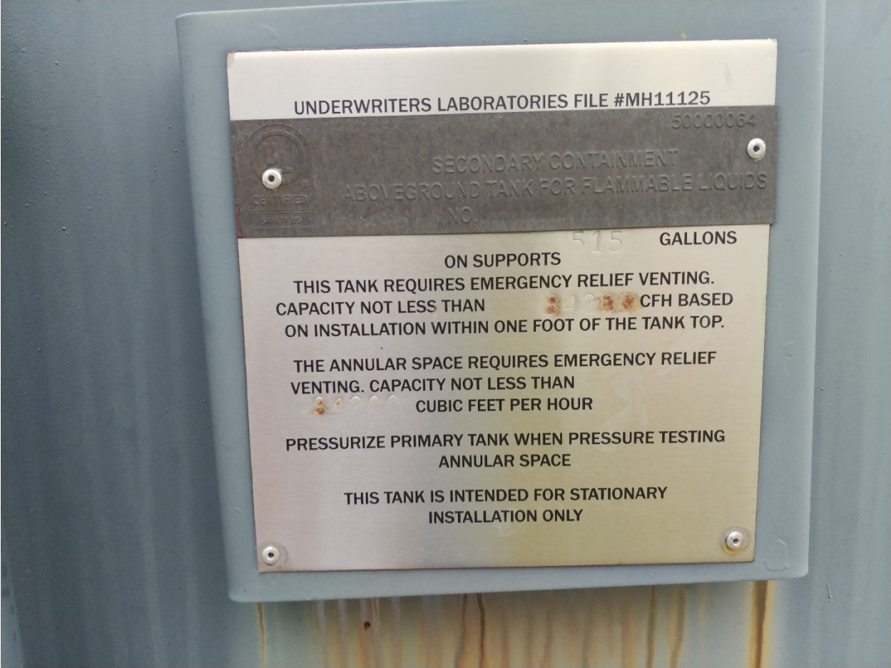
unused tank with double wall containment
